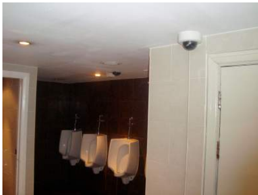
Pic. 2 – CCTV cameras inside men's washroom over urinals
